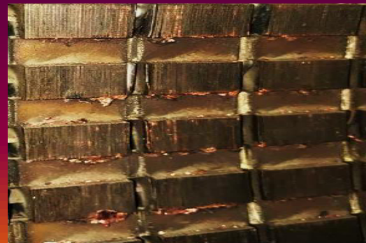
Rotor Rubbing failure
