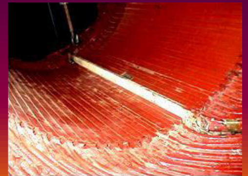
PD signs of failure
